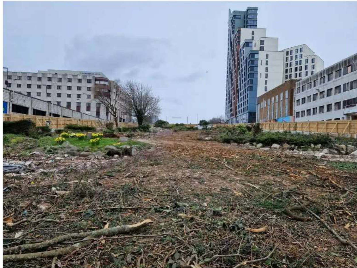
📷 The scene on Wednesday morning after the trees were felled. Photograph: Courtesy of Straw - Save the Trees Armada Way
